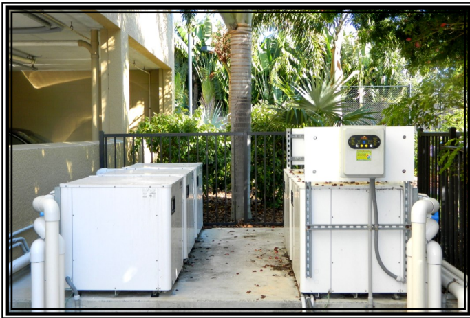
Pool heaters installed at Riva Del Lago.
